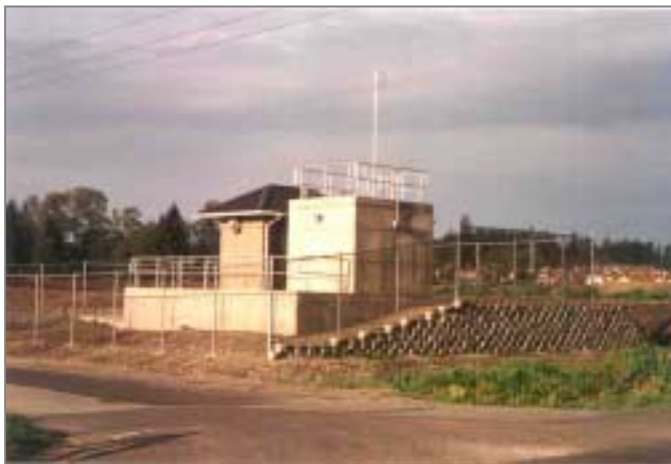
Morgan Creek Drainage Pump Station
