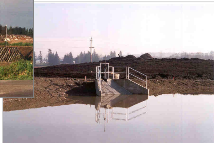
Remote Pump Station Intake Located in Retention Pond
