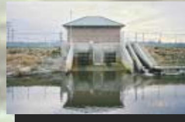
Photo No. 3 - View to the East. Showing Pump Station Outlet.
